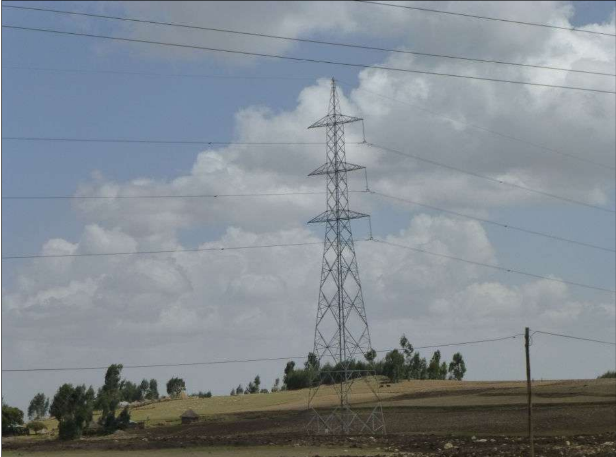
Figure 38 Pylon and 230 kV Line at the Project Site
